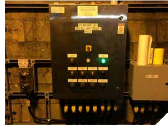
Mounted PLC control panel monitors the gear spray activity
