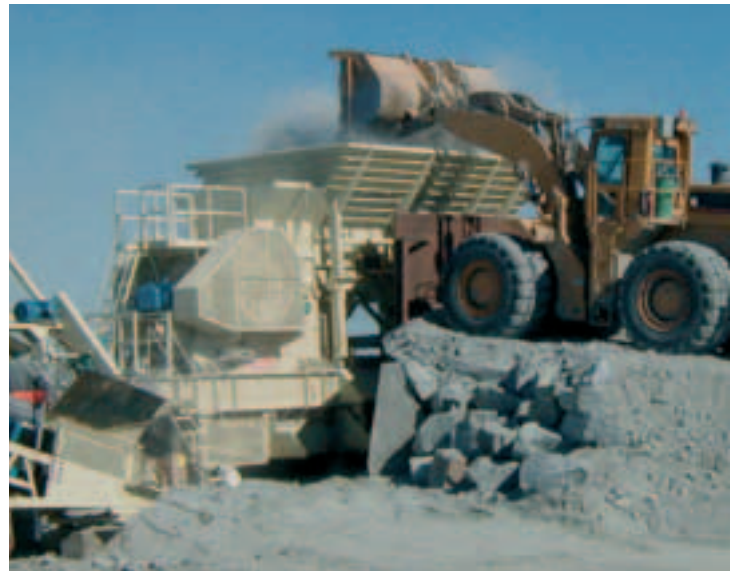
Mobile crushing with the NW125.
