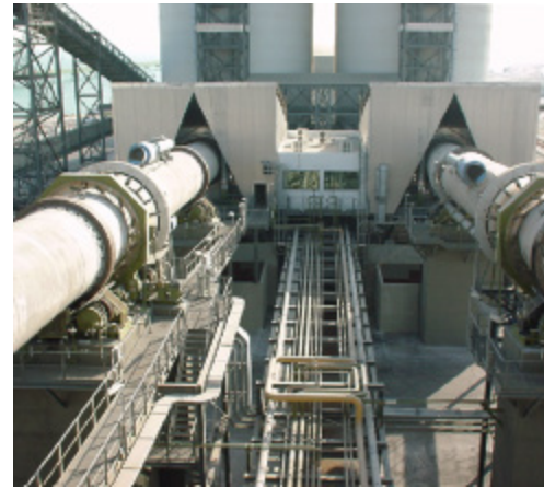
Two 250,000 MPTY Rotary kiln coke calciners
