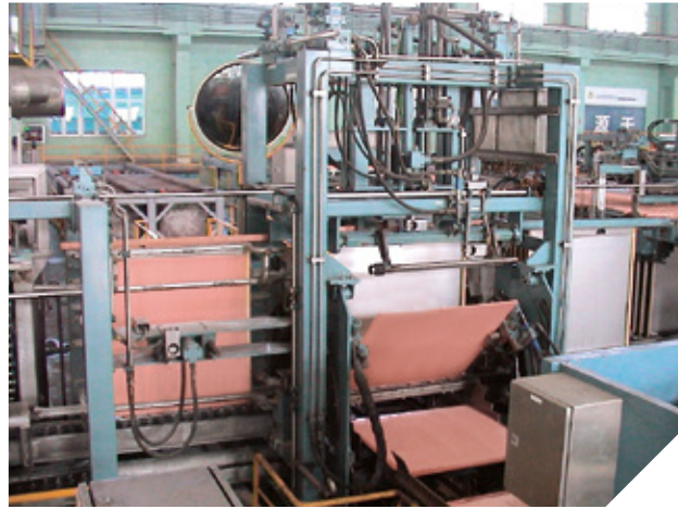
Cathode stripping machine in operation.
