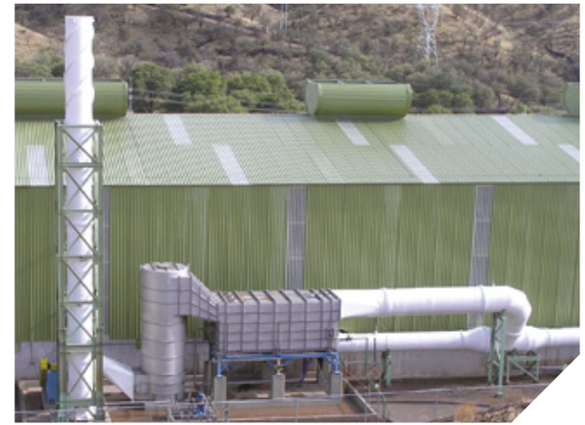
Off-gas scrubber captures tankhouse acid mists.
