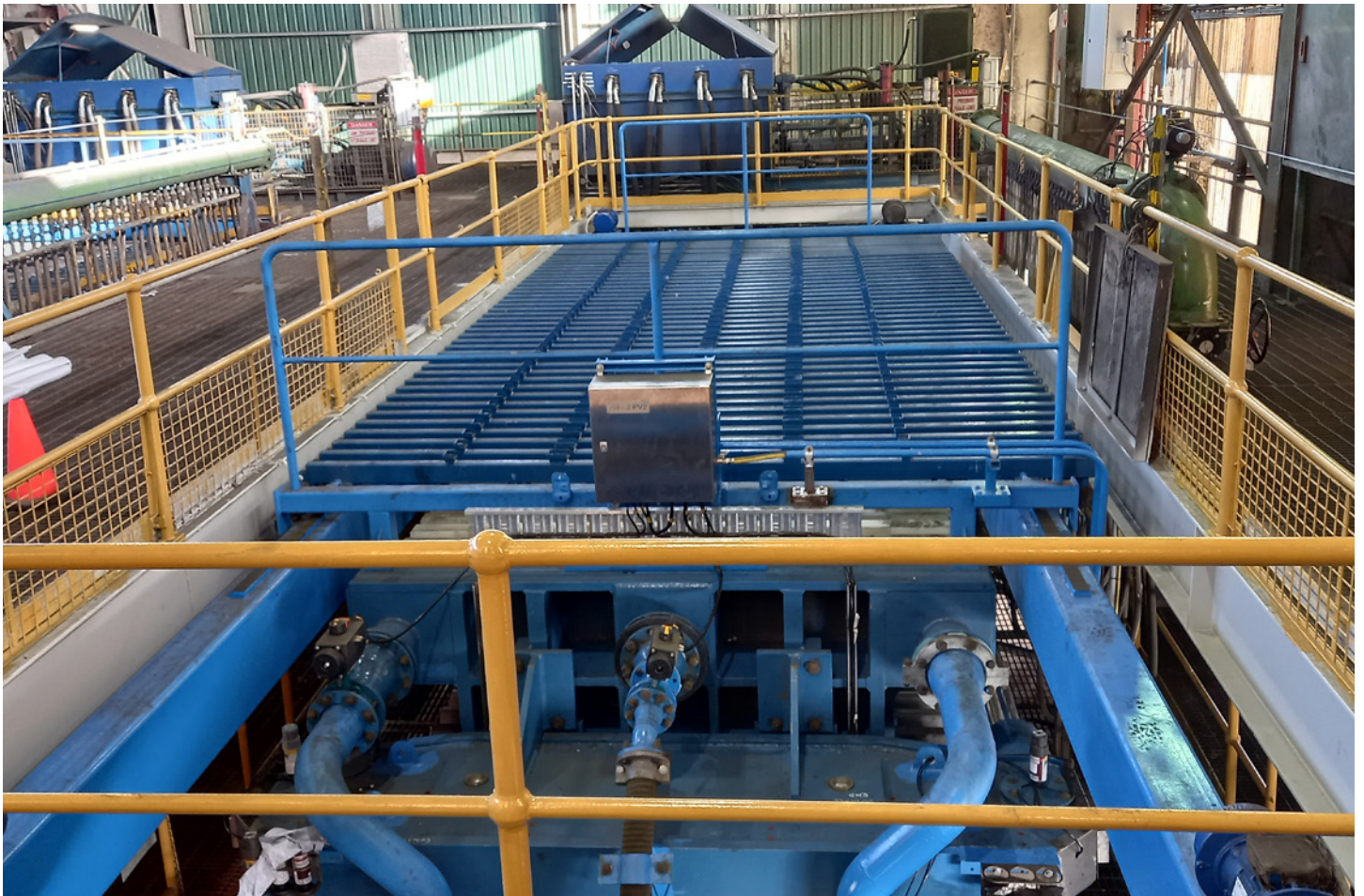
Completed VPA upgrade, back to OEM specifications, now delivering 30%+ throughput increase
