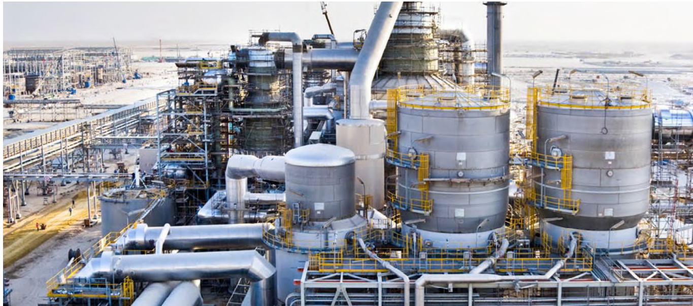
Outotec has strong expertise in fluidized bed technologies and the engineering and delivery of chemical plants, such as sulfuric acid plants. The company is the market leader in both areas.
