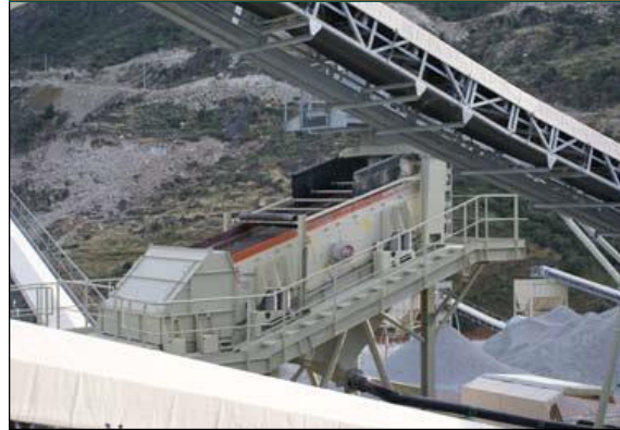
Screens and feeders
