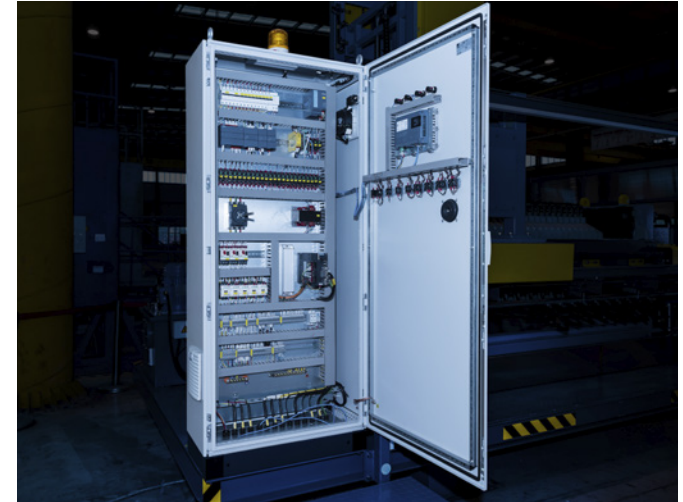
Siemens automation system and HMI
