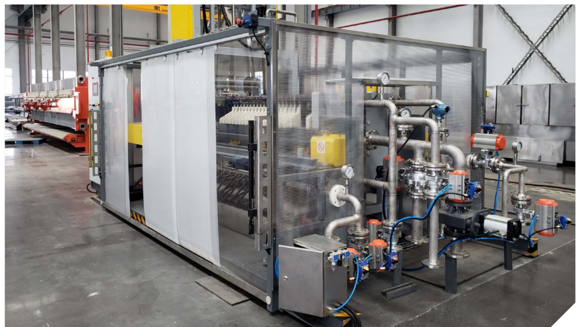
Head piping with valves and instruments
