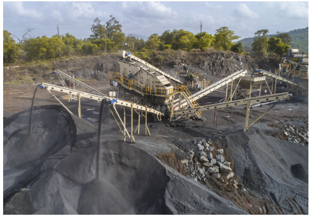
KTN Infra in Mumbai, India
