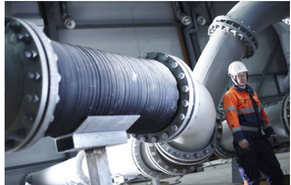
Metso slurry pipe system
